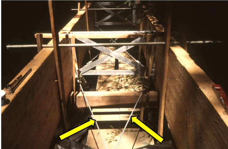
Photo 16.40 - Sway Brace Rods Attached to Diaphragms
